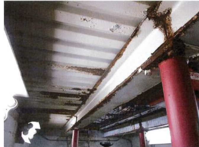
Corrosion at mechanics access basement
