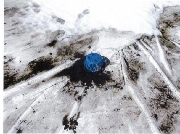
Loose roof membrane, sitting water and dirt
