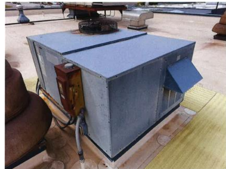
1983 Paint Booth & Body Shop Exhaust Equipment
