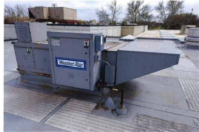
2002 Tire Room Ventilation Equipment
